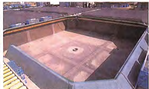
A square type tank (6m x 6m). A drain is located in the center.
